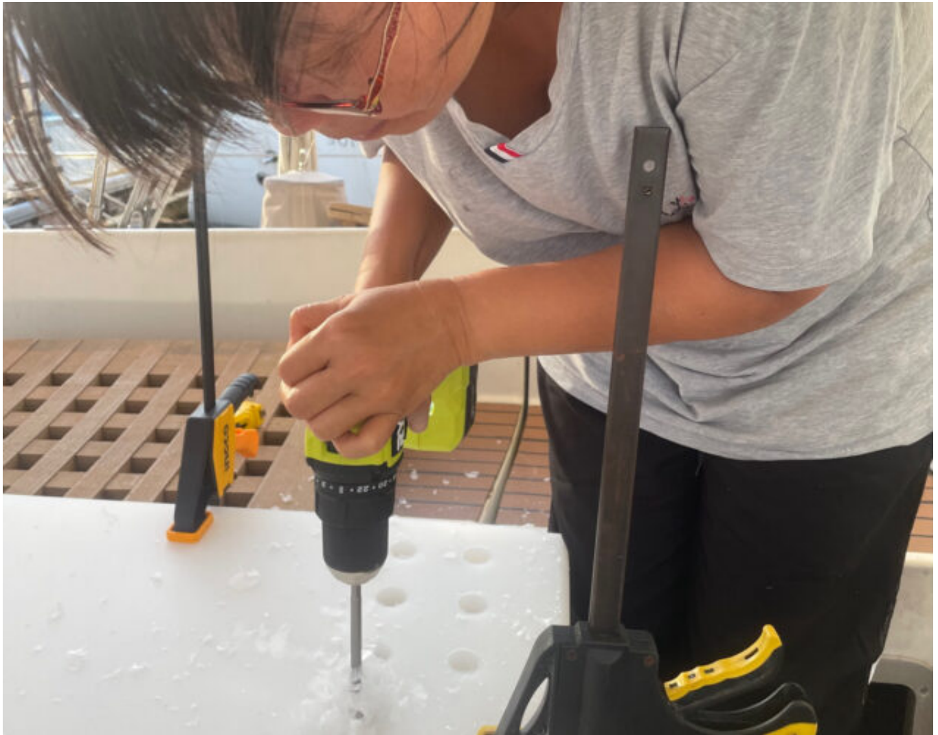
Debra drilling one of the hundreds of drainage/weight-reducing holes in the new grates.
