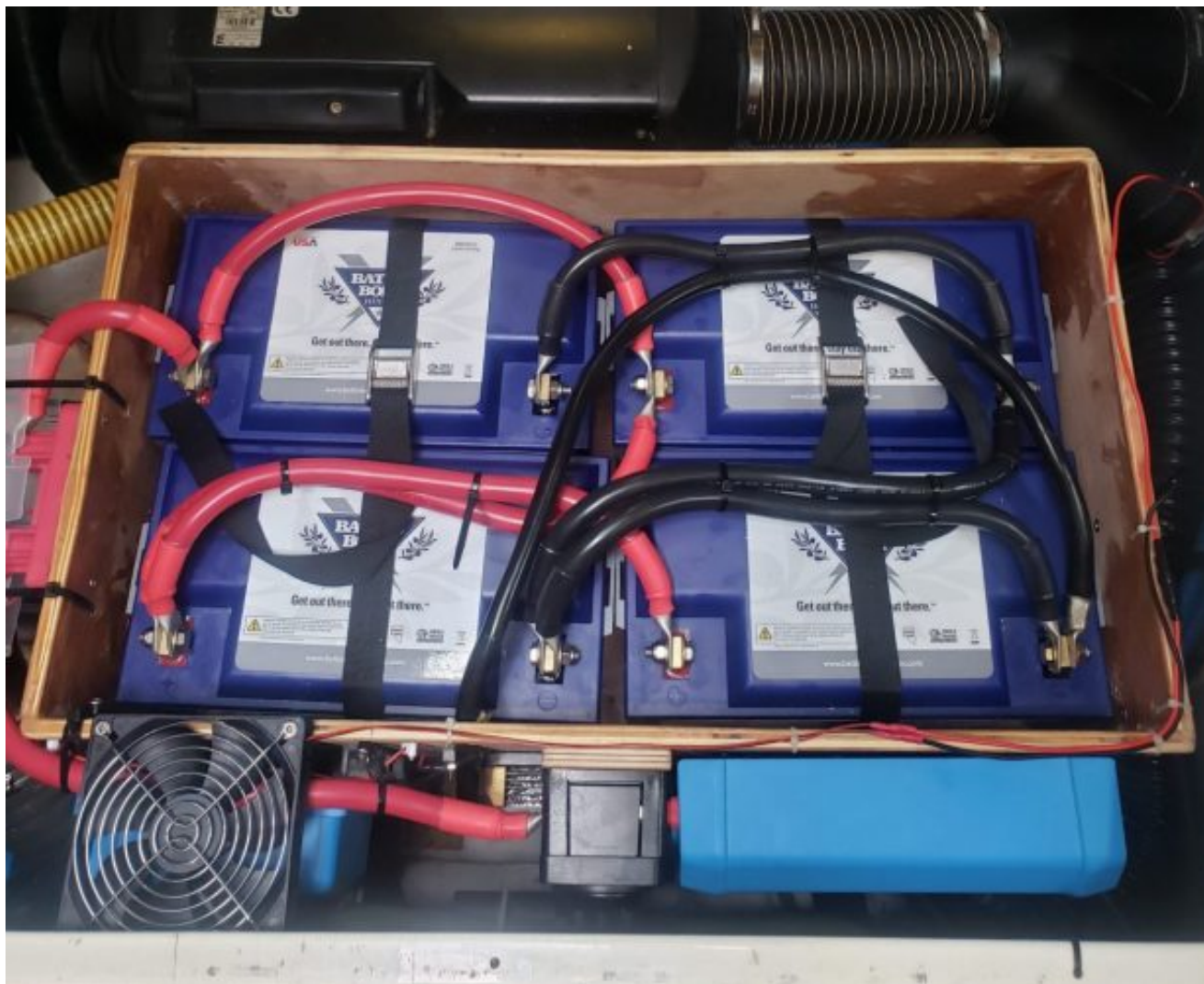
New LiFePO4 batteries ready to go
