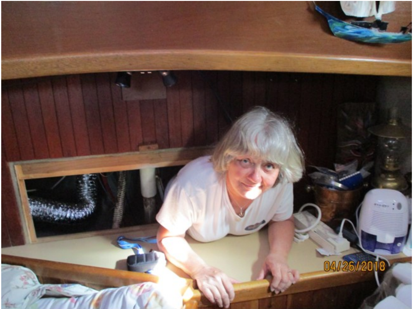
Tight spot, contains newly installed electronic equipment.
